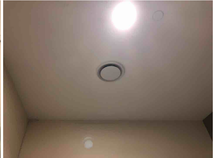
Internal Bedroom - No openable Windows. Mechanical ventilation believed to be compliant at time of construction. Exemption applies under section 22 of the Healthy Homes Standard.
