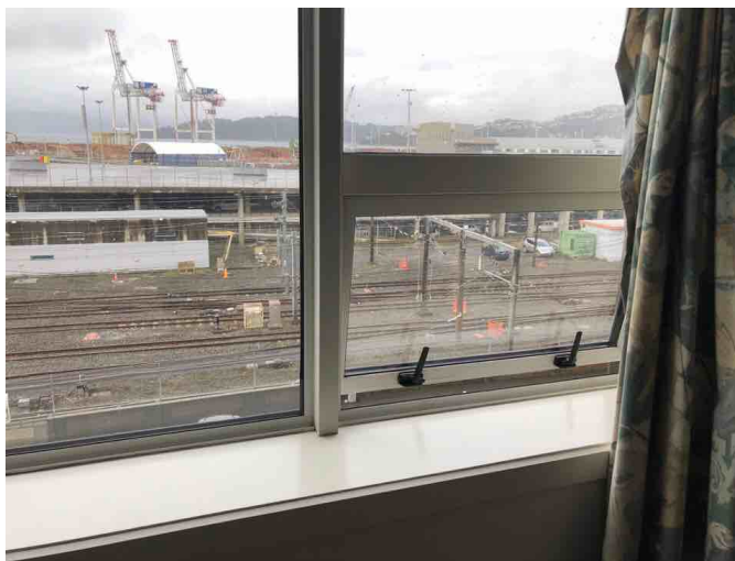
Openable windows x2@ - 0.79m x 0.43m. The Minimum ventilation requirement to meet Healthy Homes Standards in this area is 0.54m 2 . These windows provides adequate ventilation being 0.70m 2 .
